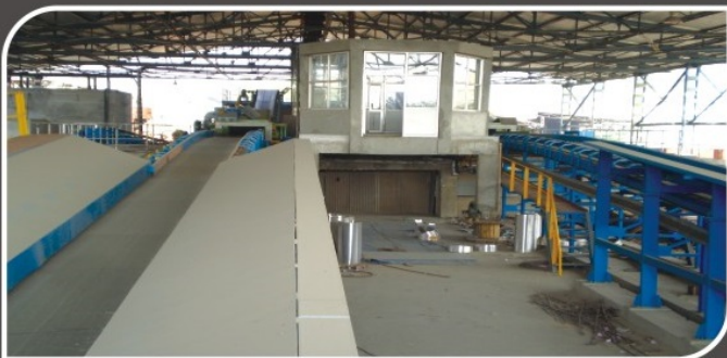
LOG CONVEYING SYSTEM
